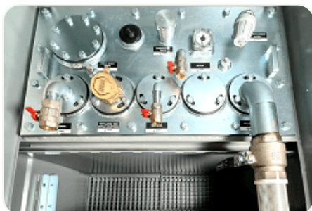
L-R fr. Back - Overfill Prevention, Pressure/vacuum relief valve & bigger flange/inspection lid.
