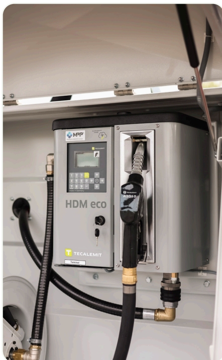
Pump and Terminal
